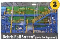
Debris Roll Screen (under OCC Separator)
