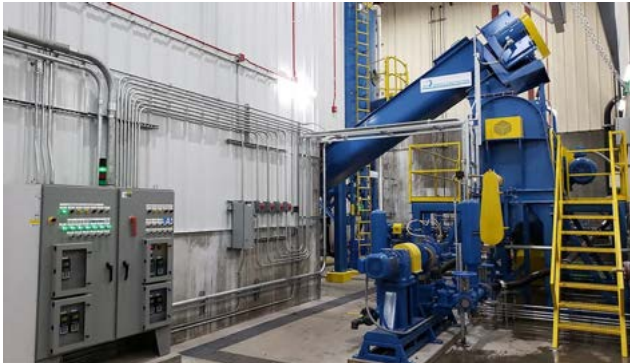
Figure 21. the THOR Turbo Separator capable of processing 30-tons of food waste per hour
